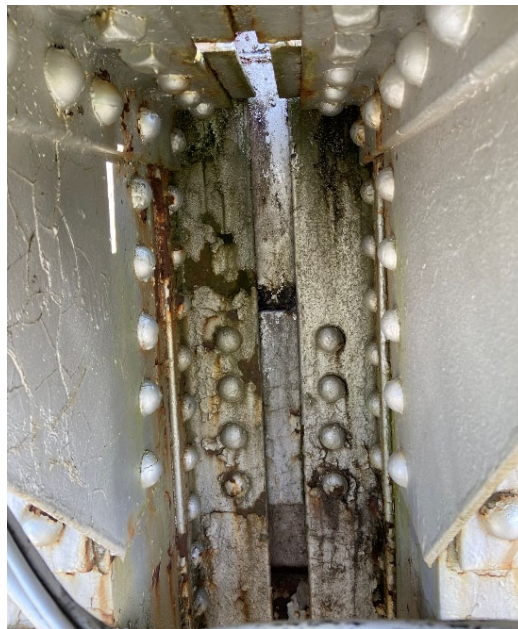
Figure 3. Light corrosion at southwest column-to-tank connection.
