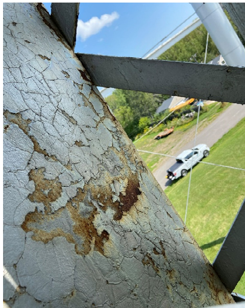
Figure 7. Cracked and flaking paint on the southwest column.
