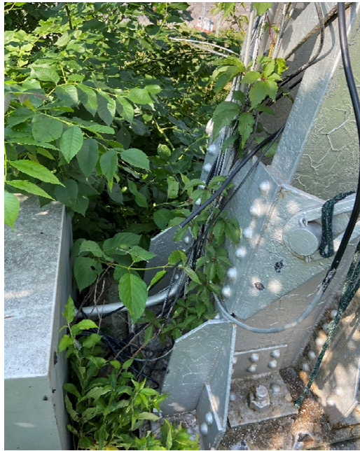
Figure 2. Dense vegetation surrounding the southeast footing.
