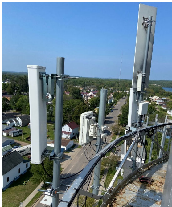
Figure 8. Several antennas attached to the walkway guardrail.
