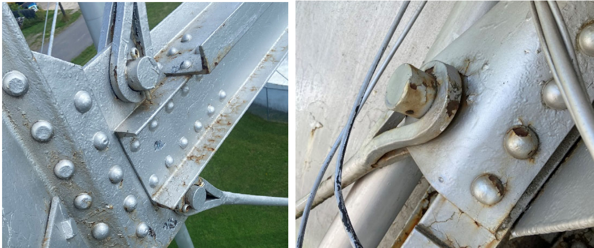
Figure 4. Typical diagonal brace clevis & cotter pin connection & connection with missing cotter pin.
