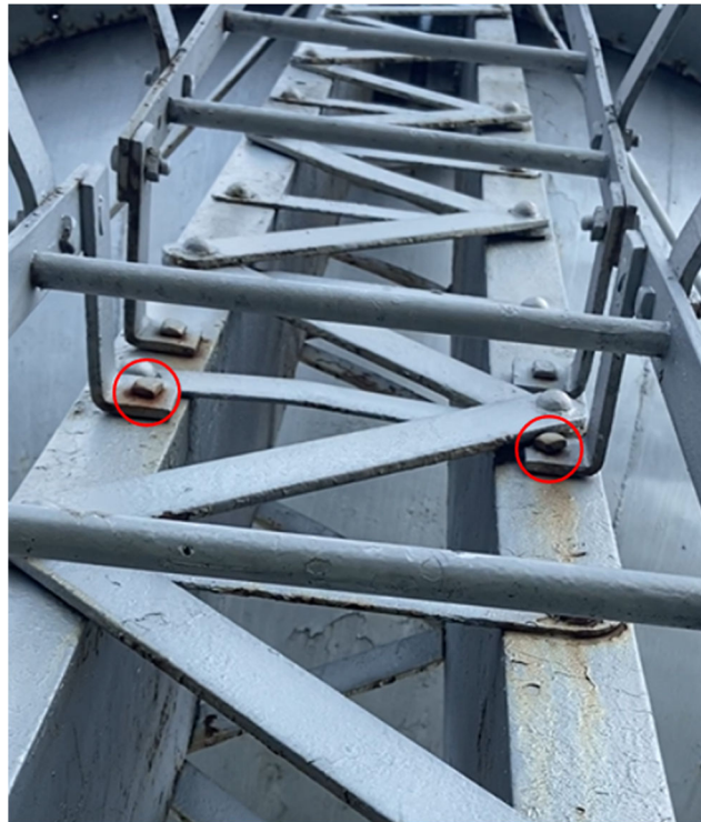
Figure 1. Loose bolts near ladder splice.
