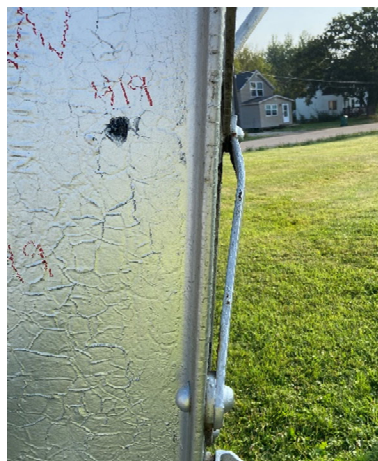
Figure 5. Buckled lace near the base of the northwest column
