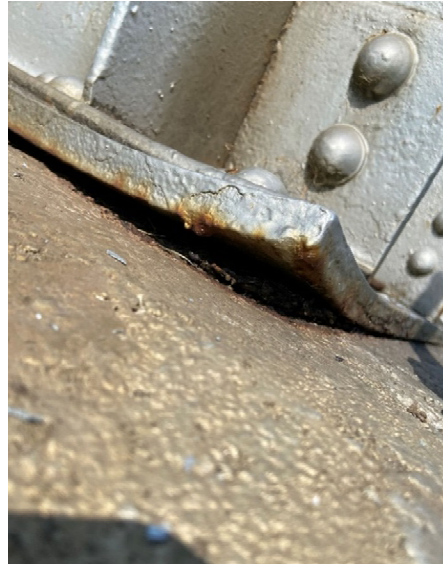
Figure 6. Bent base plate corner on the northwest column.
