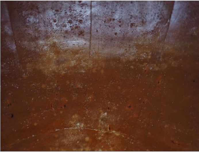
Lower sidewall after washout
