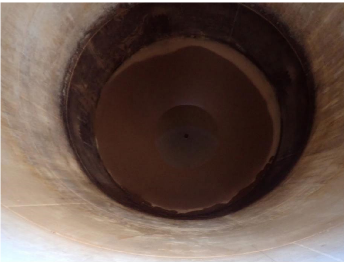
View of wet interior before washout
