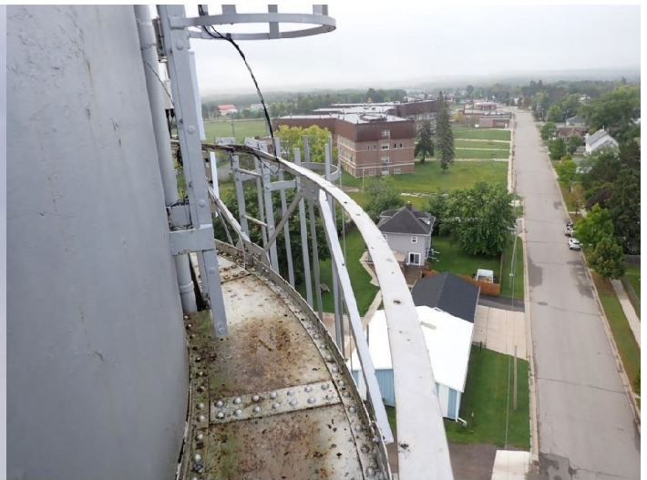
Catwalk platform and ladder
