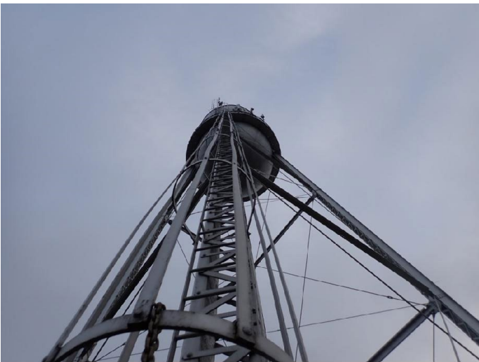
Tank leg ladder
