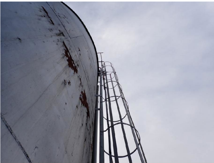
Sidewall access ladder
