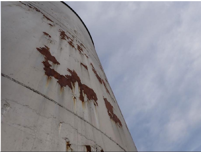
Sidewall and corrosion
