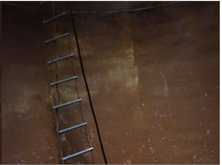
Sidewall after washout
