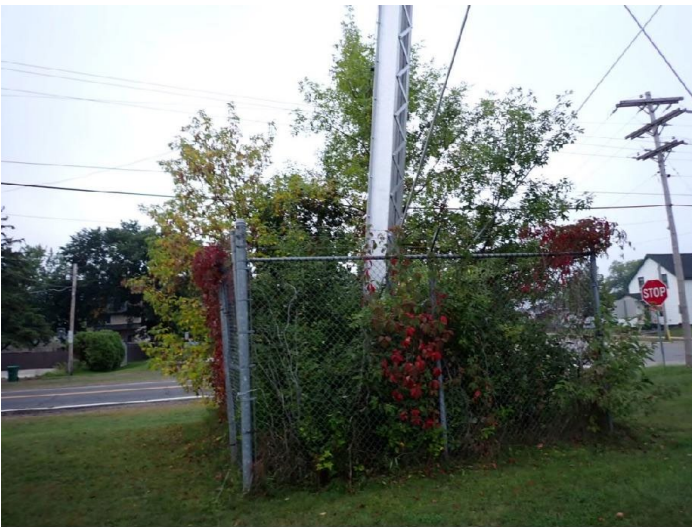
Tank leg surrounded by vegetation
